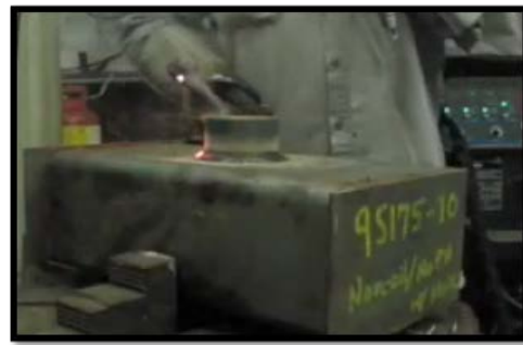
Figure 2: No Flame After Welding Phosphate Coated Fitting
